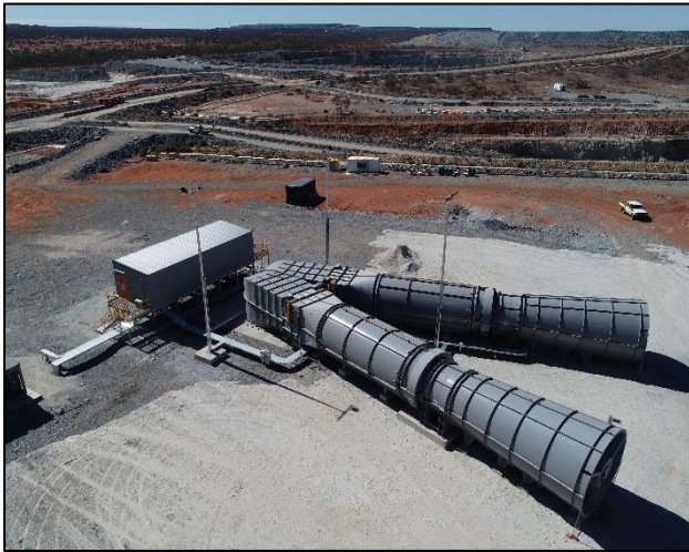
Figure 3: Primary underground ventilation
