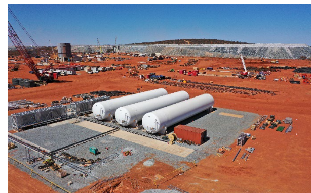
Figure 24: LNG storage installation
