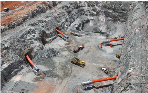
Figure 3: Initial ventilation fans installed and commissioned
