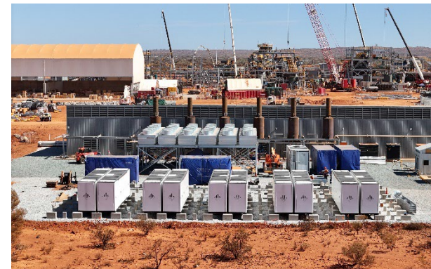
Figure 22: Power station engine hall
